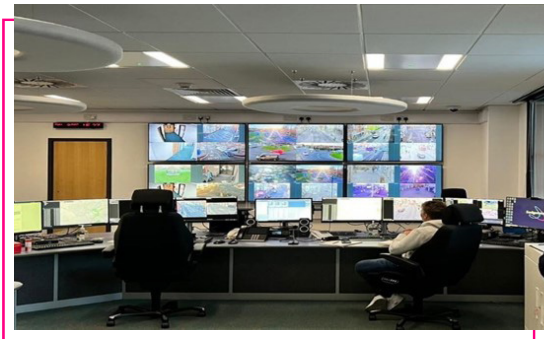
Sedgemoor District Council CCTV Monitoring Office
