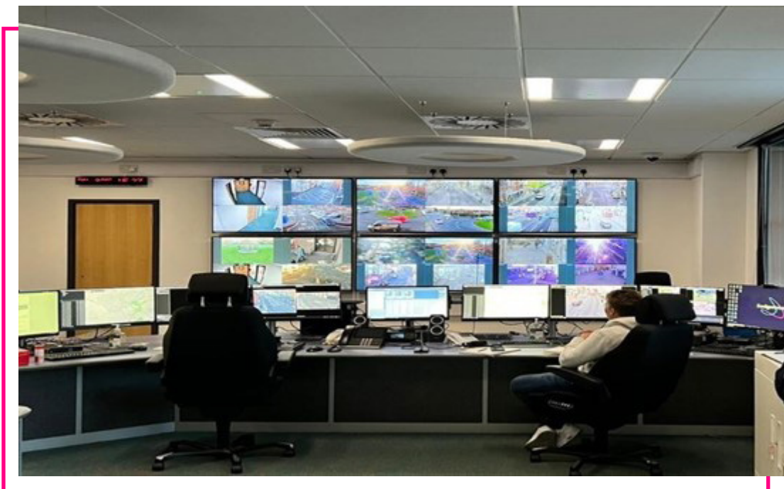
Sedgemoor District Council CCTV Monitoring Office
